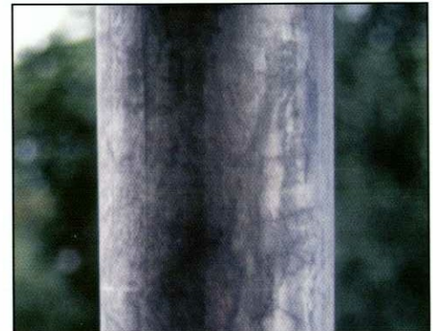
Mottled appearance when light grey pure zinc is surrounded by dark grey zinc-iron alloys developed, for example where reaction is greater at grain boundaries and locally allows the full thickness of coating to convert to zinc-iron alloy.
