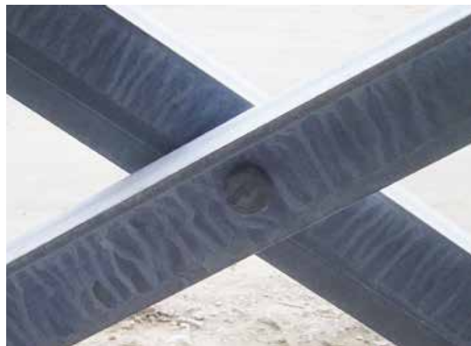
Fig 1. Wet storage stain formed on galvanized surface
