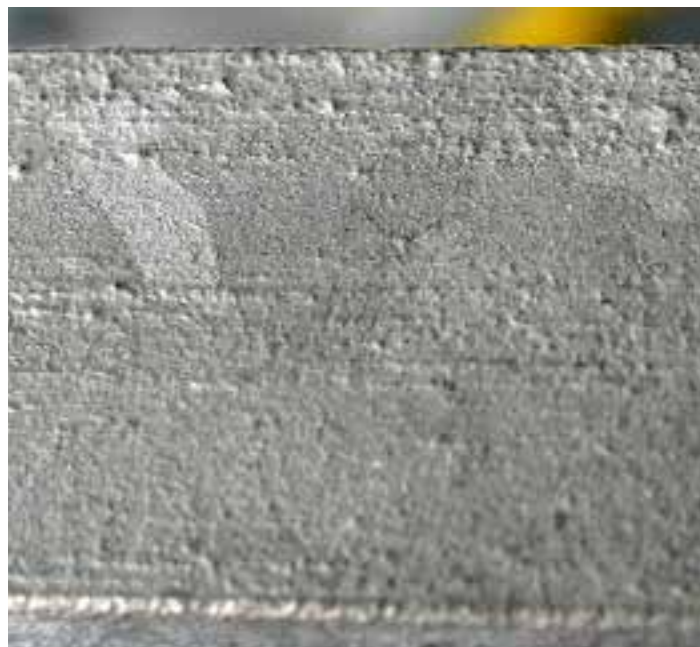
Fig 1. Uneven coating due to variable surface steel chemistry
