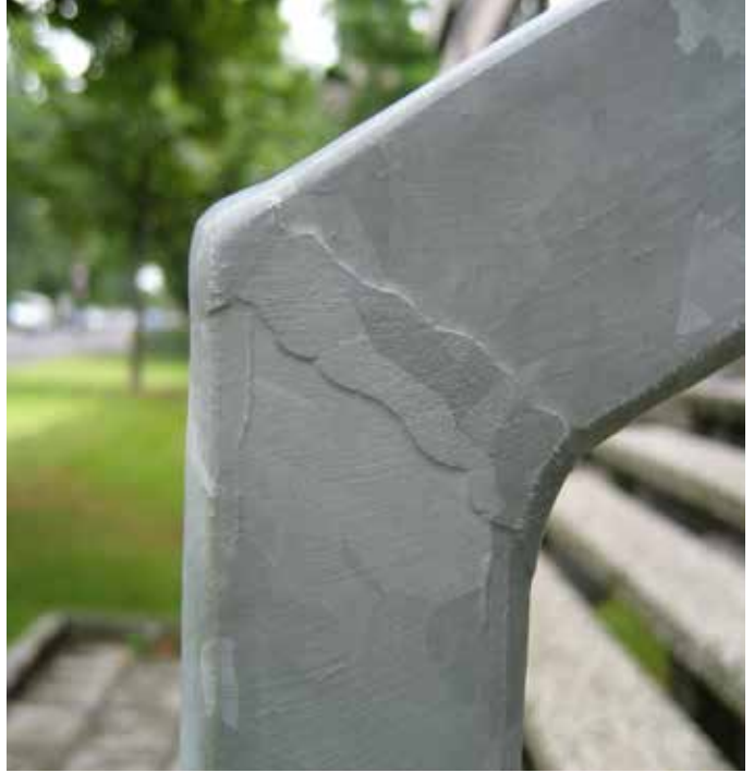
Fig 4. A weld that was ground flush prior to galvanizing. The high silicone content of the weld metal has then led to a thicker coating forming locally
