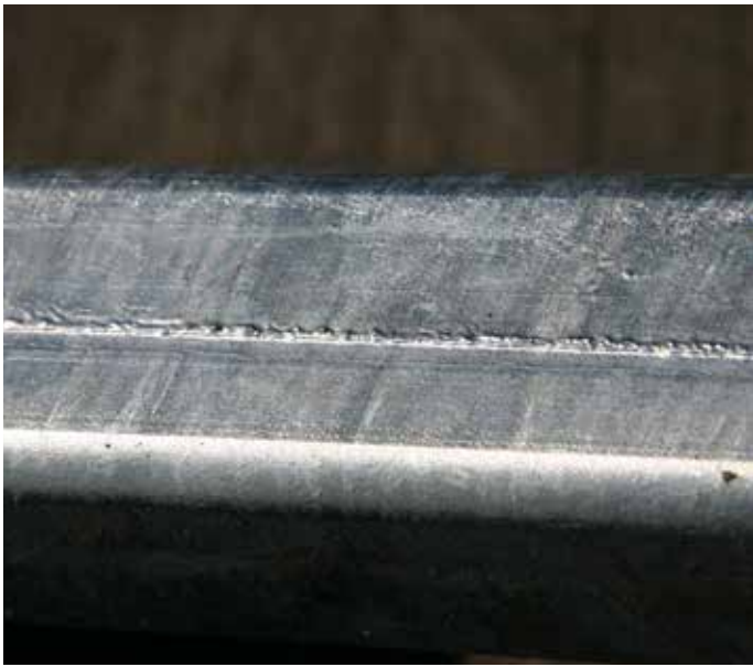
Fig 3. Build-up of the galvanized coating along the weld seam of a box section
