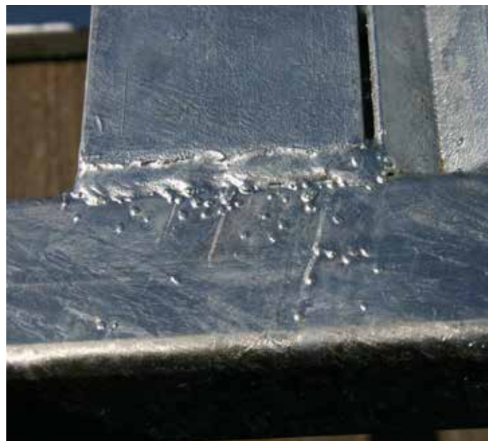
Fig 2. Area of weld spatter not removed prior to galvanizing
